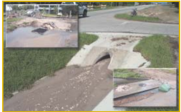
Pollutant Discharge in Storm Drains
